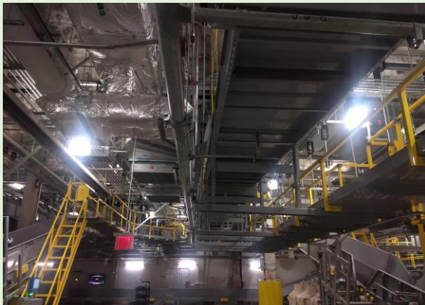
ENERGY CONSERVATION & MECHANICAL
