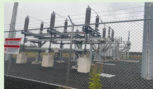
SOLAR SUBSTATION INSPECTION
